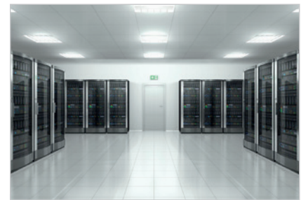
Fig.: Constant processes and highly sensitive applications such as data centres, are based on RCM monitoring.
